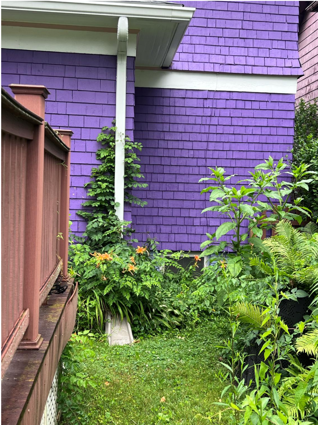
Exhibit "C" Rear of House Location of Condenser
