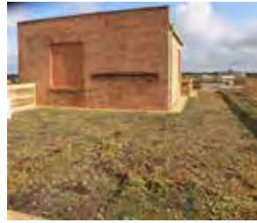
Toledo School for the Arts started a Storm Water collection roof.
